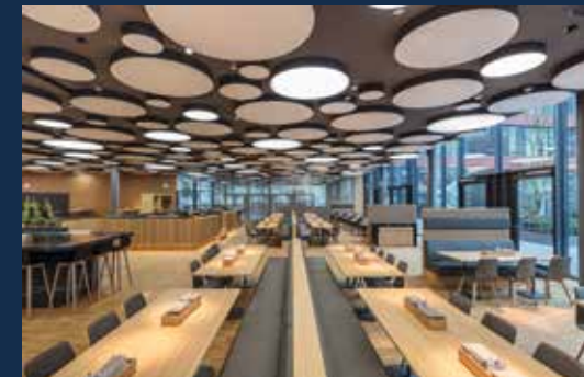
Via the building management system: In the canteen, hold-open systems also help control the air-conditioning.
