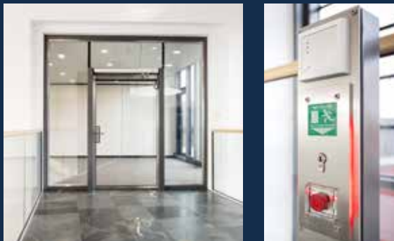
Complex door technology, fine-framed and centrally controllable. The LED background lighting of the door control unit (right) shows the “locked” door mode.
